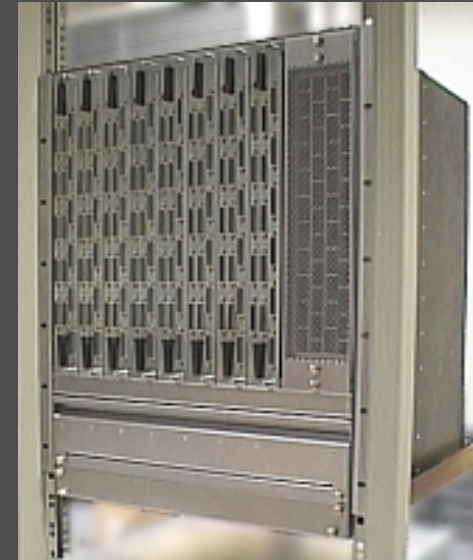
128 way Switch Chassis
